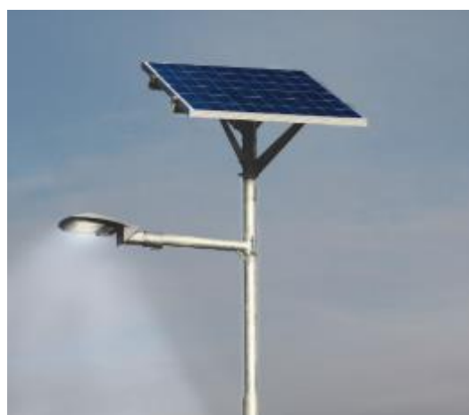
Fig. 4.15.2. Solar panel fuelled public lighting.
