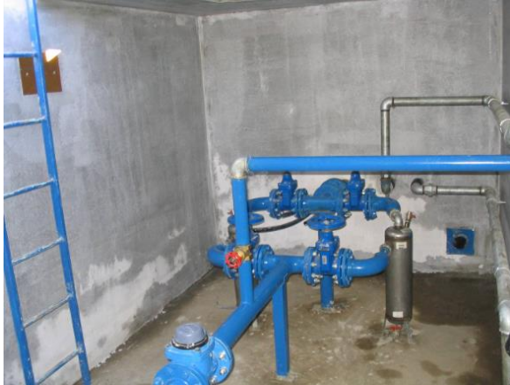
Fig. 6.3. Groundwater well providing heat.
